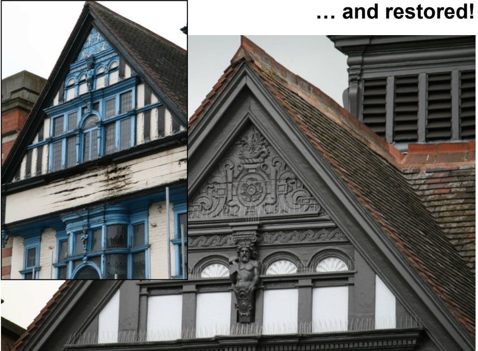
Detail of the gable end facing East Gates, before and after the recent restoration
